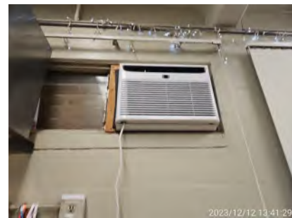
Air conditioning in kitchen
