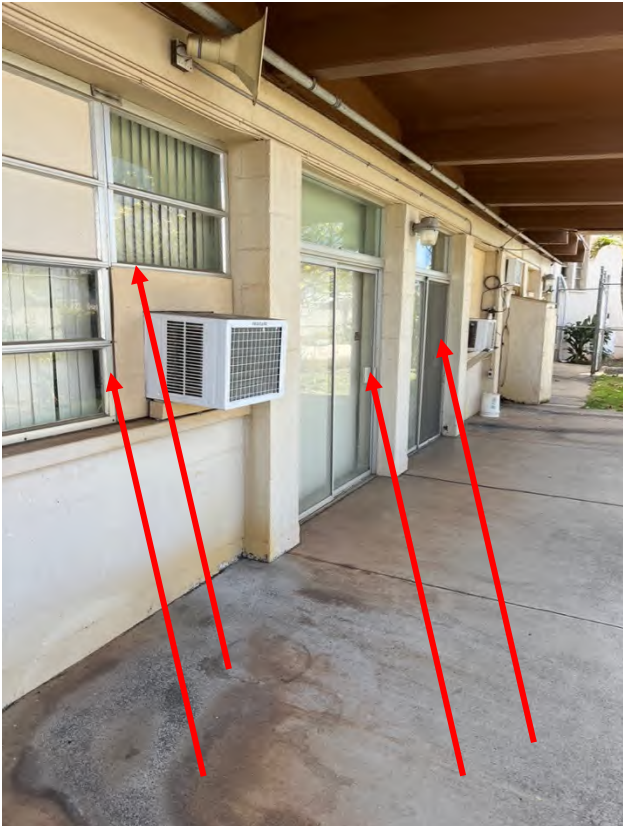
Asbestos detected in gray caulking painted off white around kitchen windows and sliding door
